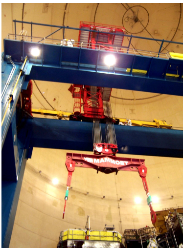
Operation in nuclear plant
