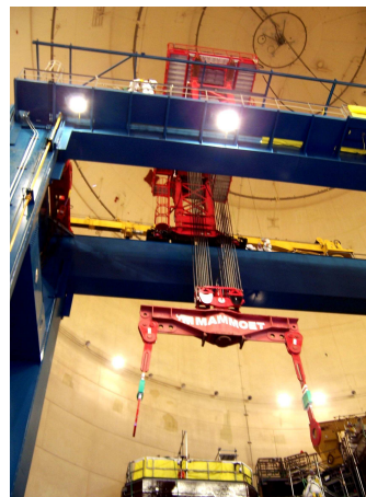
Containerized gantry (red) on main gantry (blue) for retracting heat exchangers in a nuclear power plant
